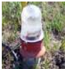
Runway Edge Lights
