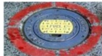
Hydrant Fueling Pit
