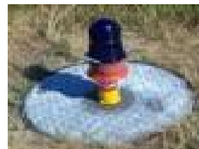
Taxiway Edge Lights
